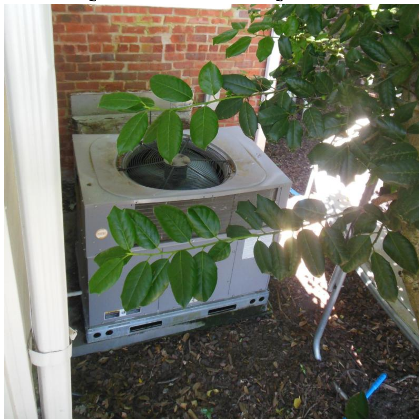
Rear House HVAC Unit (Existing - 'To Be Relocated')
